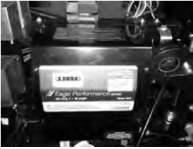
On-board battery charger located under hood
