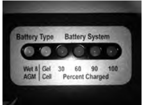
Battery Charger meter
