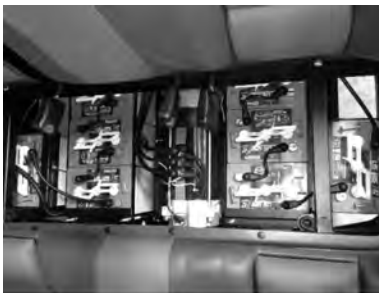
Batteries located under seat
